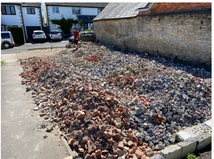
Some of the hardcore and rubble that has been moved and broken down to form the base for the extended parking area at the rear of the property - 10th August 2022
